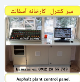
Asphalt plant control panel
