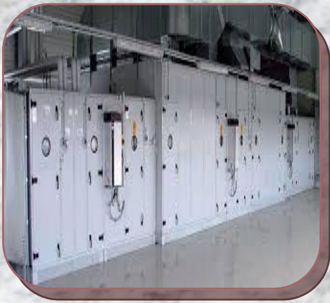
AIR HANDLING UNIT
